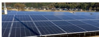
Facilities supplying renewable energy to the head office building
